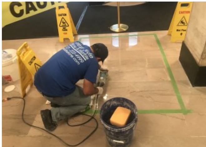
West Side Stone and Marble, a vendor participant of the CU Grow program, at work in a Columbia University building.
